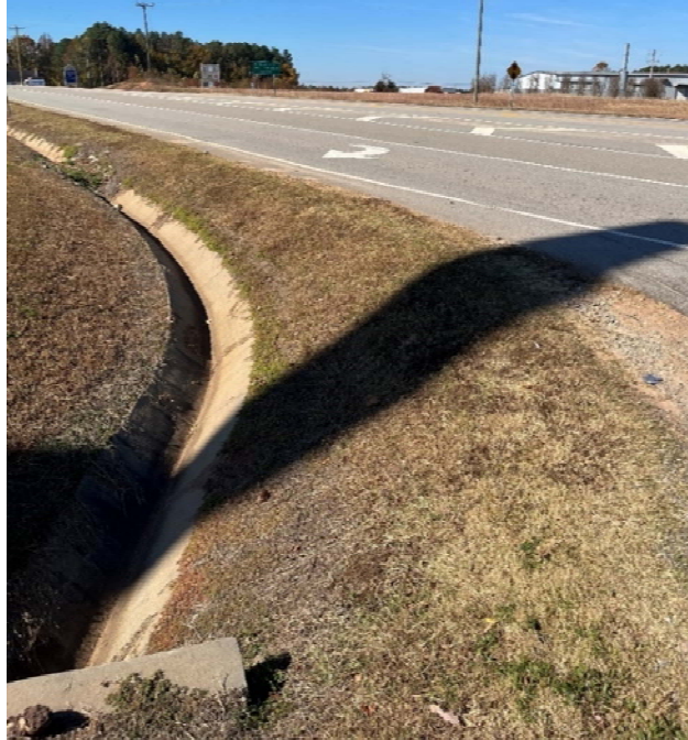
Figure 8 : Drainage along North Mecklenburg Avenue (Photo: Toole Design)
