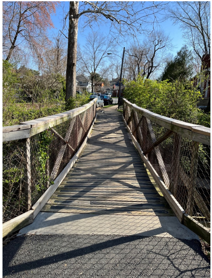
Figure 9. Sag on Bridge No. 9007
